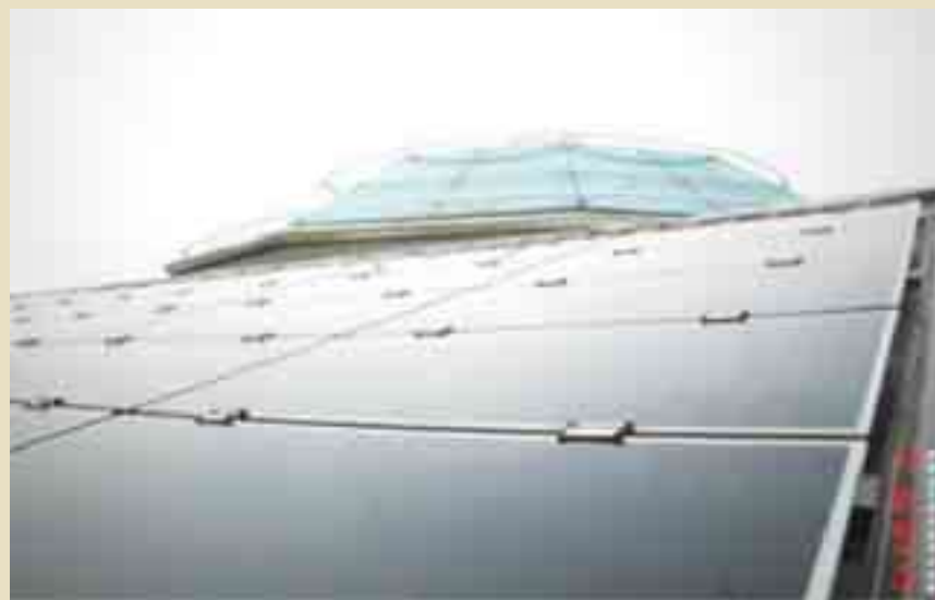
Photovoltaic solar panels on rooftop.
