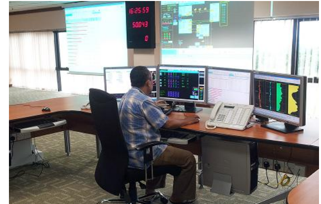
BACKUP CONTROL CENTRE (BCC)
